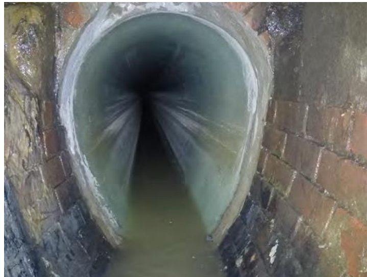
Figure 20 – Rehabilitation works on the 130 year old Upper Hobson Bay main sewer. (Source: Interflow 2019)
